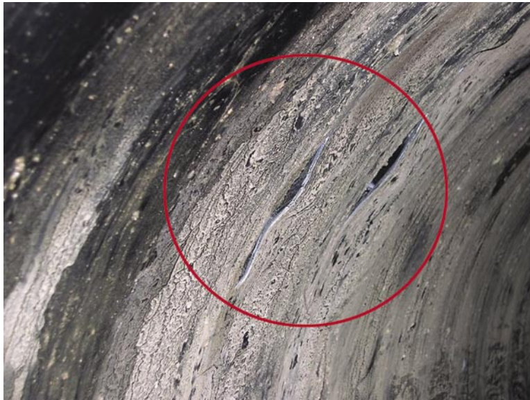
Project 10, Homer, showing cracks in pipe wall above spring line
