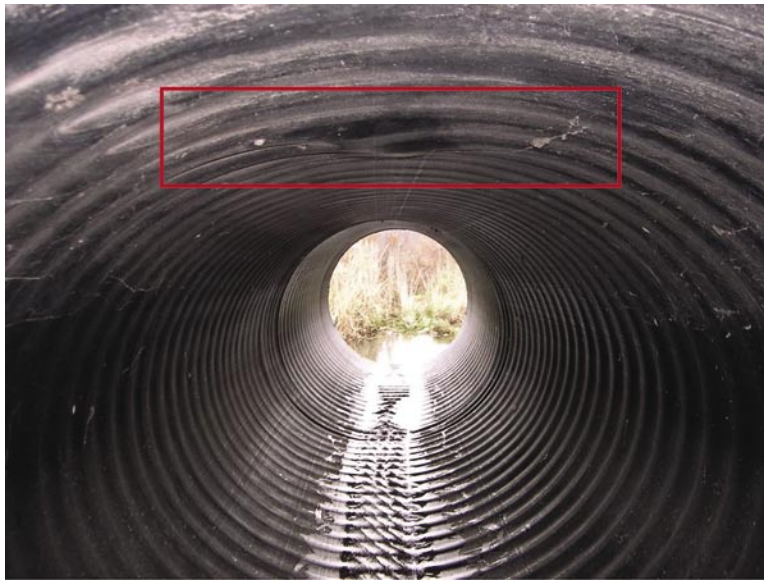
Project 10, Homer, showing bulge in crown
