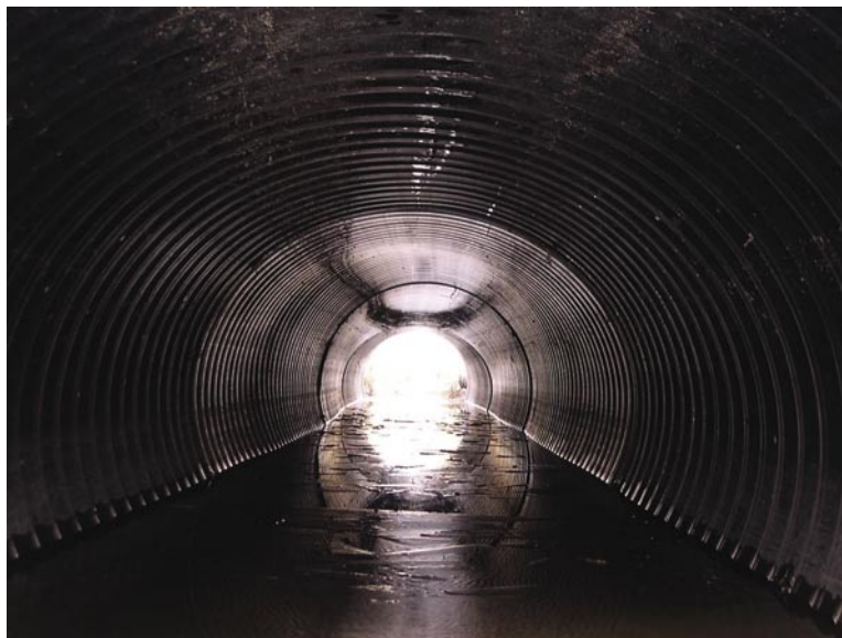
Video Image on Project 2, Dola showing vertical deflection and racking
