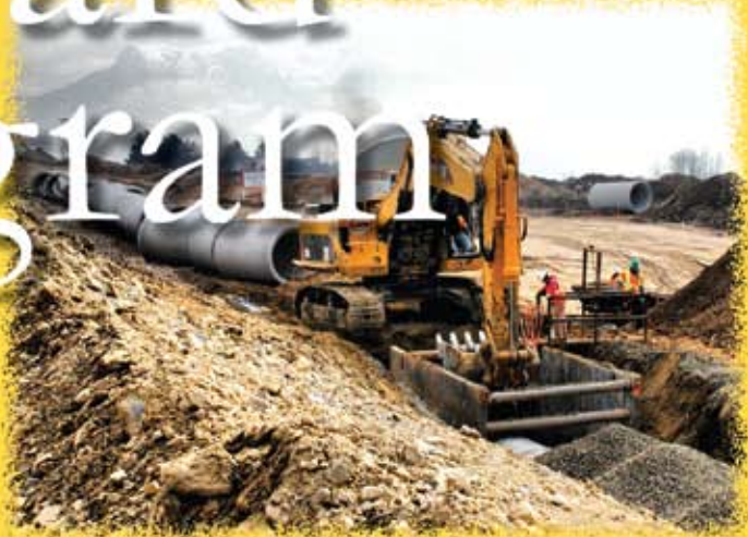
SR-92 Highway Drainage Pipe, Lehi, UT Photo: Mountain States Concrete Pipe Association
