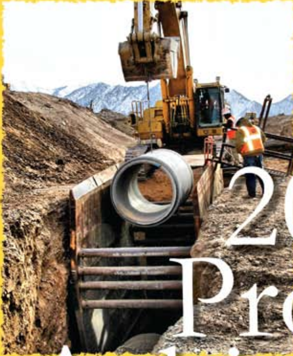
SR-92 Highway Drainage Pipe, Lehi, UT Photo: Mountain States Concrete Pipe Association
