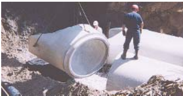
Reinforced precast concrete pipe used as end-of-life solution for failed corrugated metal pipe culvert.
